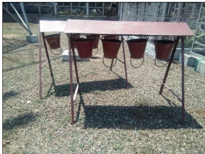
Photographs of the fire extinguisher provided within unit
